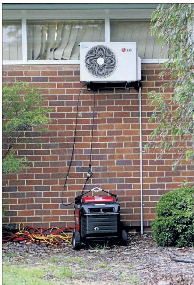
POWER-LESS: A portable generator in use at Peakhurst South Public School after a power outage lasting several days from Sunday February 9. Picture: John Veage
